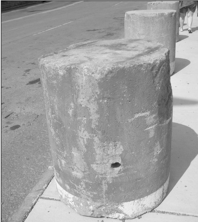
UGLY BOLLARDS: City Hall threatened to take me to court because city sidewalks were not wide enough at my property. At my expense, I doubled their width, costing me $11,000. Unbelievably, the city placed half-ton eyesore bollards on those same city sidewalks, restricting the flow of pedestrians and giving an unkempt appearance near the entrance of the State Park.
